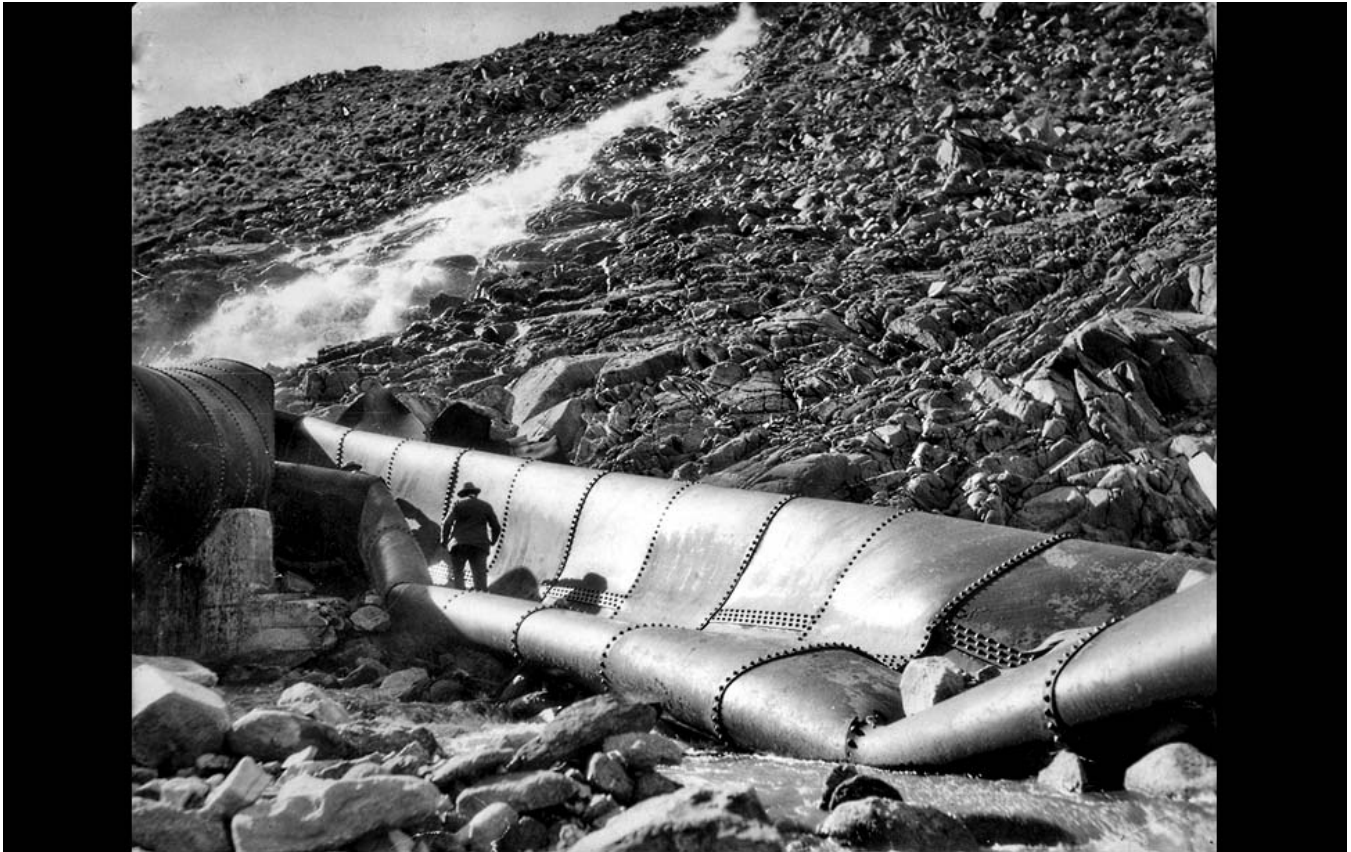
Damaged aqueduct. (Photo courtesy of Rich McCutchan)
