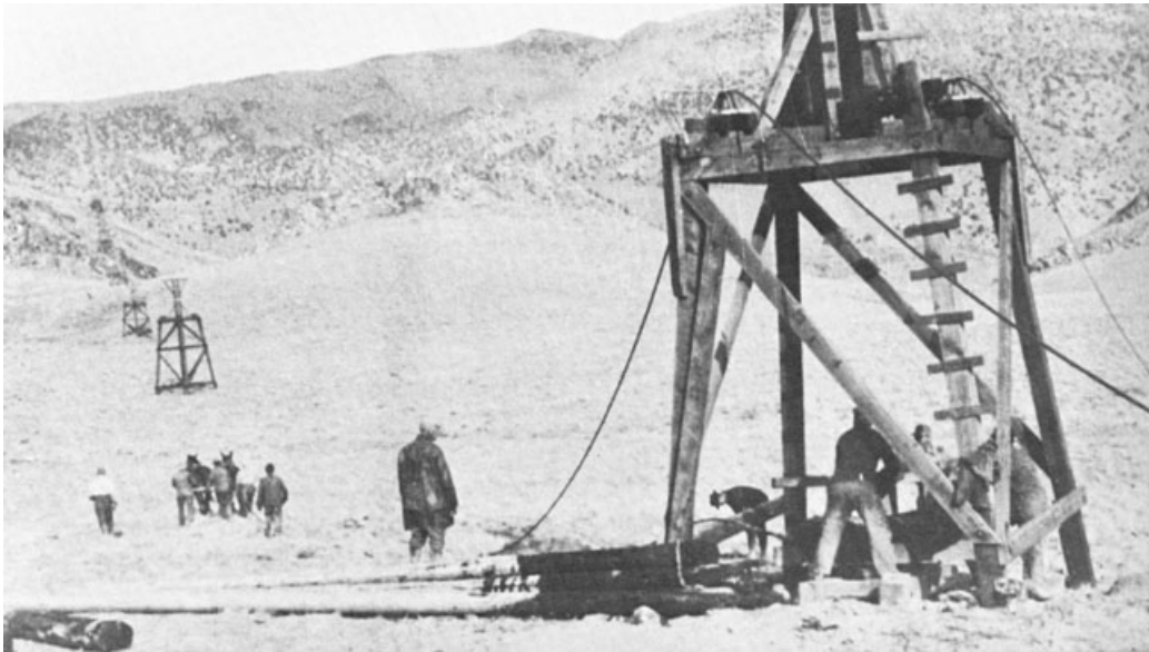
This view looking west from the Saline Valley depicts the construction during 1912 of the tram towers.
